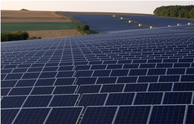
Exhibit 12: Solar Photovoltaic panel
